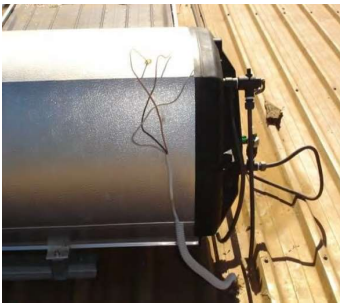
Unterminated live cable shorted to frame of HWS bushed. Possibility of complete roof being energised energised
