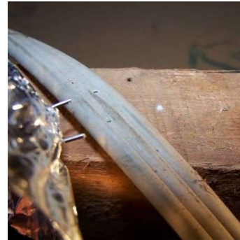
Metal staple pierced cable Foil insulation may be
