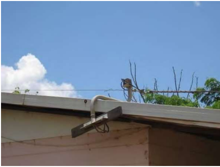
Service riser collapsed due to rotted fascia. Supply still connected energised
